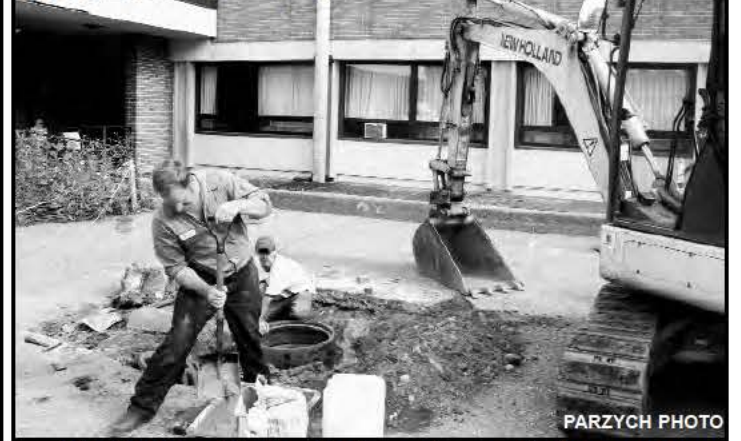
John Conley, of Conley Services, mixes mortar for employee Doug Smith who is mortaring bricks supporting a manhole cover ring at the Farren in Montague City, in preparation for paving by Felton Construction.
