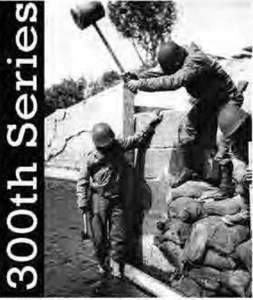
300th Combat Engineer Battalion repairing the under piling of a bridge destroyed by enemy fire along the Carentan - Cherbourg Road in France - June 30, 1944.
