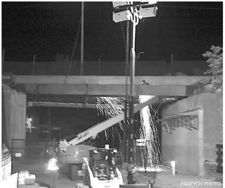
The night shift cuts beams on the Turners bridge approach over the bike path.
