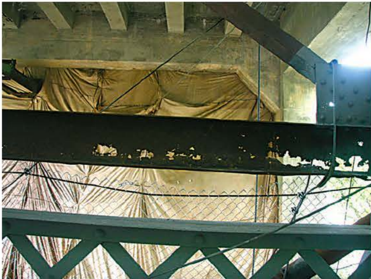
Renovation of the Gill-Montague Bridge comes none too soon, by the look of this carrying beam, on the Gill side of the structure. A canvas tarp isolates a section of the bridge's understorey to enable painting and shot blasting to continue.
