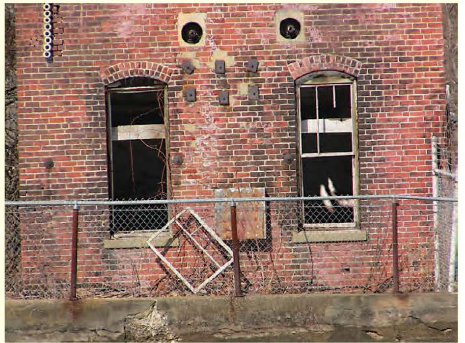
Many of the old mill buildings along the Power Canal have fallen into disrepair.
