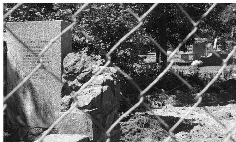
Chainlink on the Park. Construction has already begun downtown, creating some less than attractive streetscapes. It's the short term price for the improvements changing the face of downtown.
