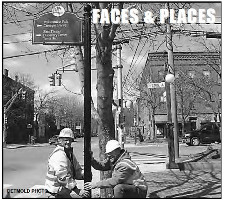
Theodore Liddell and Jim Lake, of Liddell Brothers, from Halifax, installed seven wayfinding signs in Turners Falls and two on Route 2, on March 24th.
