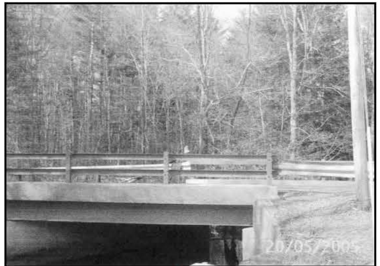
After the Gill Highway crew tackled the job, the bridge looks good as new.
