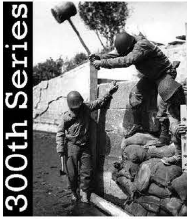
300th Series 300th Combat Engineer Battalion repairing the under piling of a bridge destroyed by enemy fire along the Carentan - Cherbourg Road in France - June 30, 1944.
