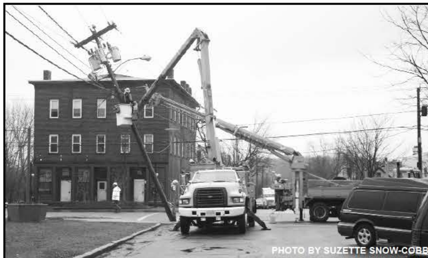
A semi taking a right on Second Street on the way to the Southworth Mill clipped the utility pole on the corner, causing widespread power outages downtown on Wednesday
