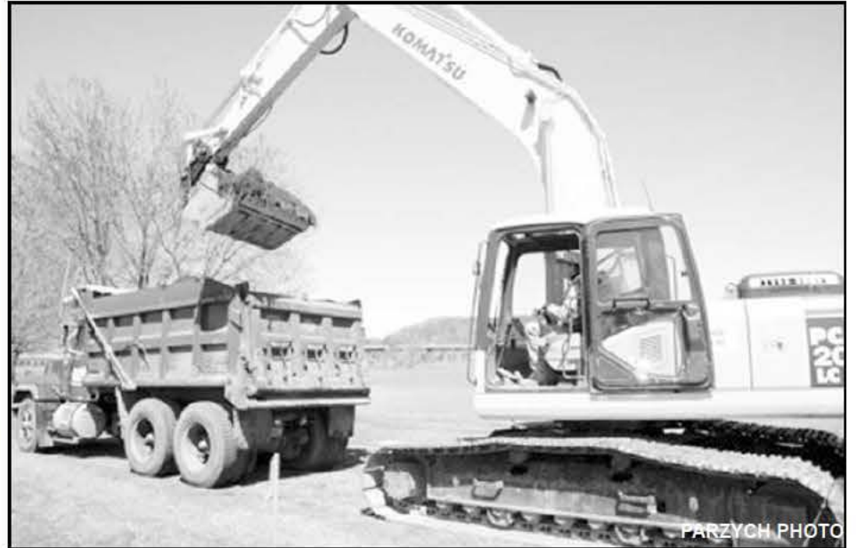
Danny Potralya, operating a Komatsu excavator, loads a Mack dump truck driven by Jim Streeter on the bike path project in Turners Falls.
