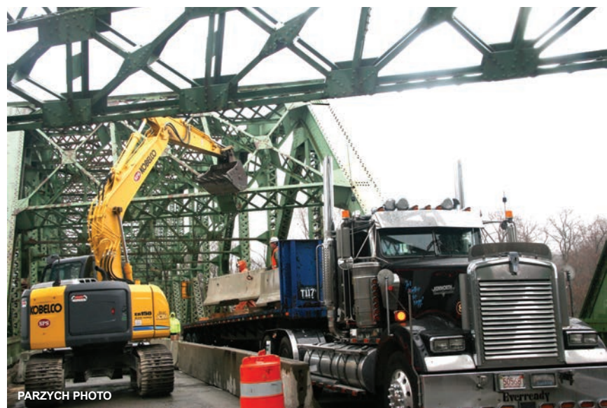
Barriers cordoned off the work area on the General Pierce Bridge last week
