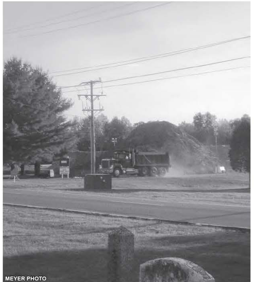
Northfield, September 6, 2010: One of thousands of truckloads FirstLight had to dredge back out of the Connecticut River.
