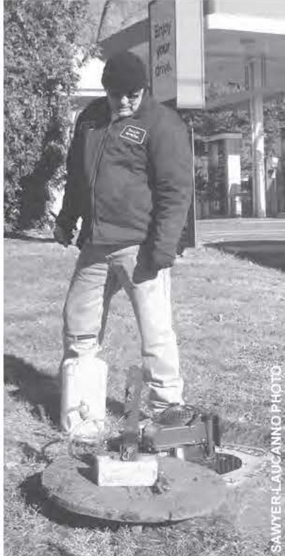
Eddie Ambo of the Gill DPW blows smoke into the sewer lines.
