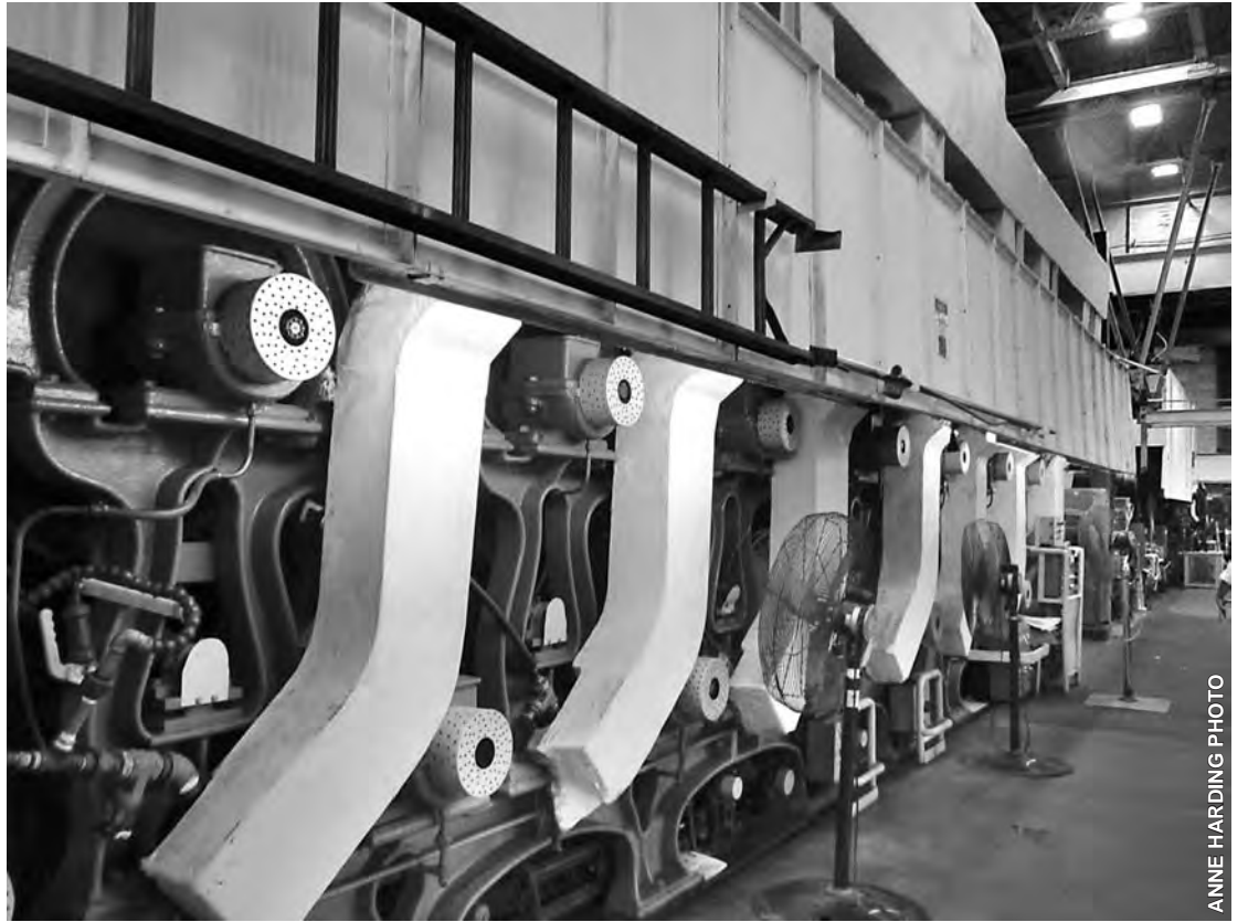
This high-heat drying system is one of the final steps in the process at the facility.
