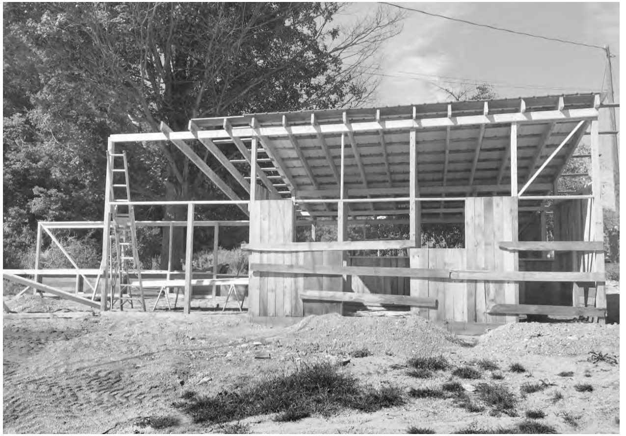
Craig Memorial Equestrian Center suffered a fire last spring that completely ruined one of the barns. While all horses escaped, the barn must be completely rebuilt. The construction is partially complete, but Roberta Bryant is still looking for donations to cover the cost.
